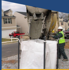
PRE-FABRICATED SACK WASHOUT
