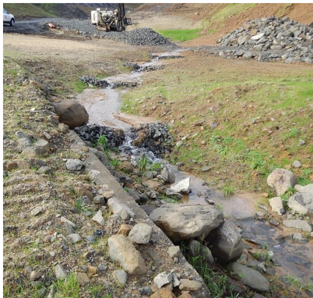
Figure 2-11 Check Dams slow runoff velocity
