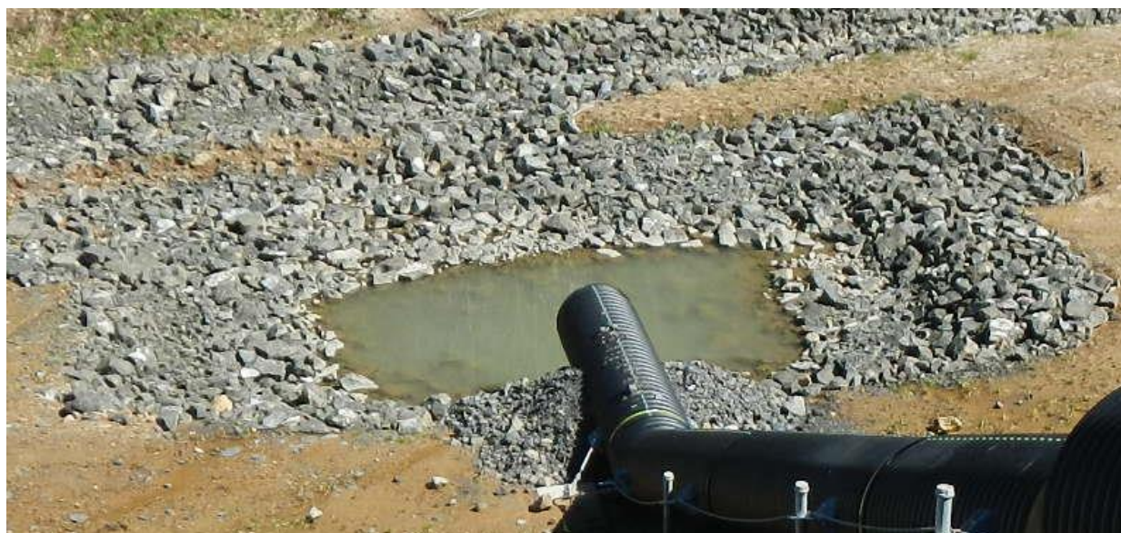
Figure 3-16 Energy Dissipater (permanent installation)
