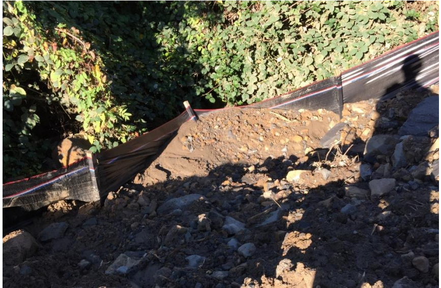
Figure 3-29 Sediment fence maintenance failure
