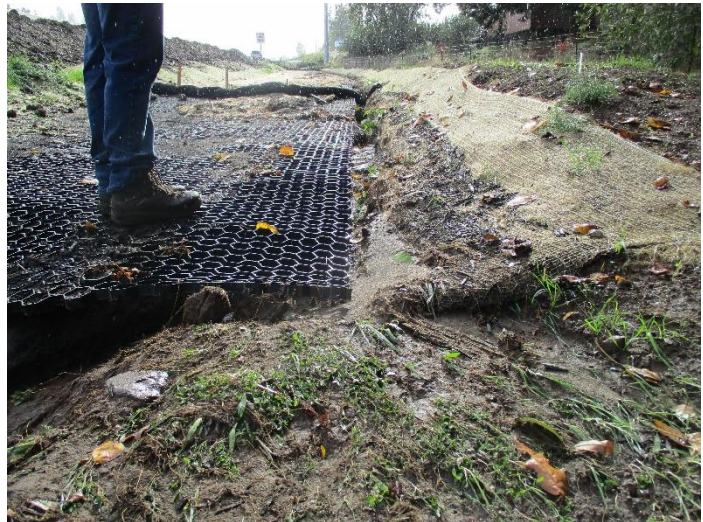
Figure 2-7 Erosion control failure at water quality facility
