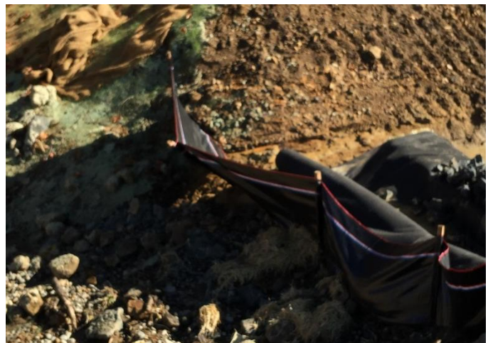
Figure 3-30 Sediment fence not embedded in ground
