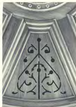
Above: Detail of ceiling medallion that once graced the 24 foot ceiling above the second floor courtroom. Below: Drawing of the proposed changes to the Circuit Courtrooms. (Courtesy Cy Stads vold, Benton County Courthouse Study, 1977).
