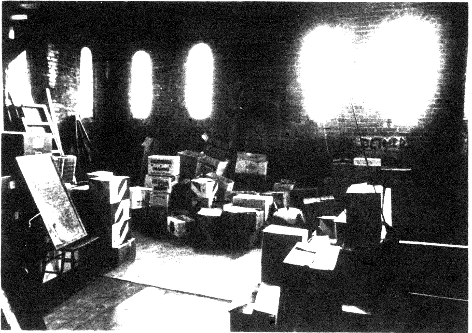
The fourth-floor attic of the Benton County Courthouse, now used for storage, would be made into a law library if plans for renovating the courthouse are carried out. The ladder at the left leads to the belltower.
