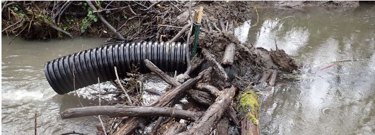
Outlet pipe of beaver pond leveler installed on Dunawi Creek to help reduce flooding of 53 rd Street.
