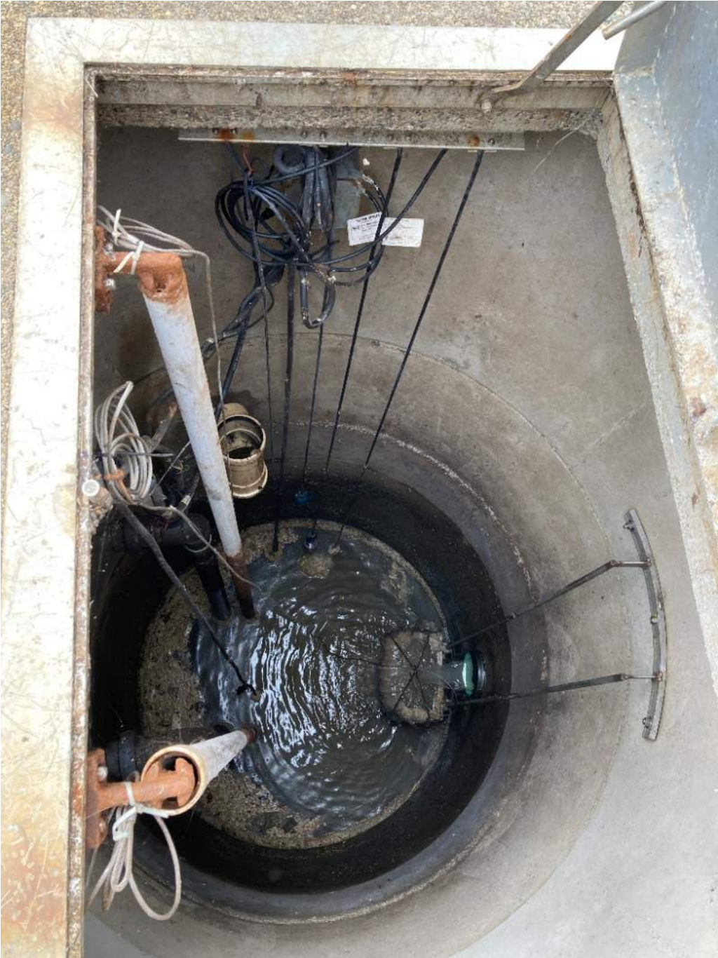
Figure 3-2 Influent Lift Station
