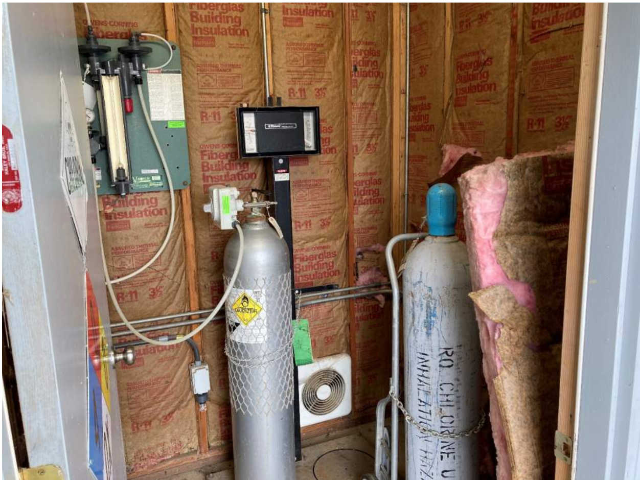
Figure 2-6 Gas Chlorination System
