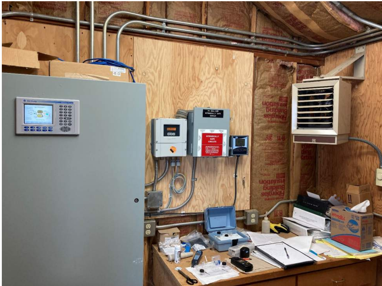
Figure 2-9 Electrical and Controls Room
