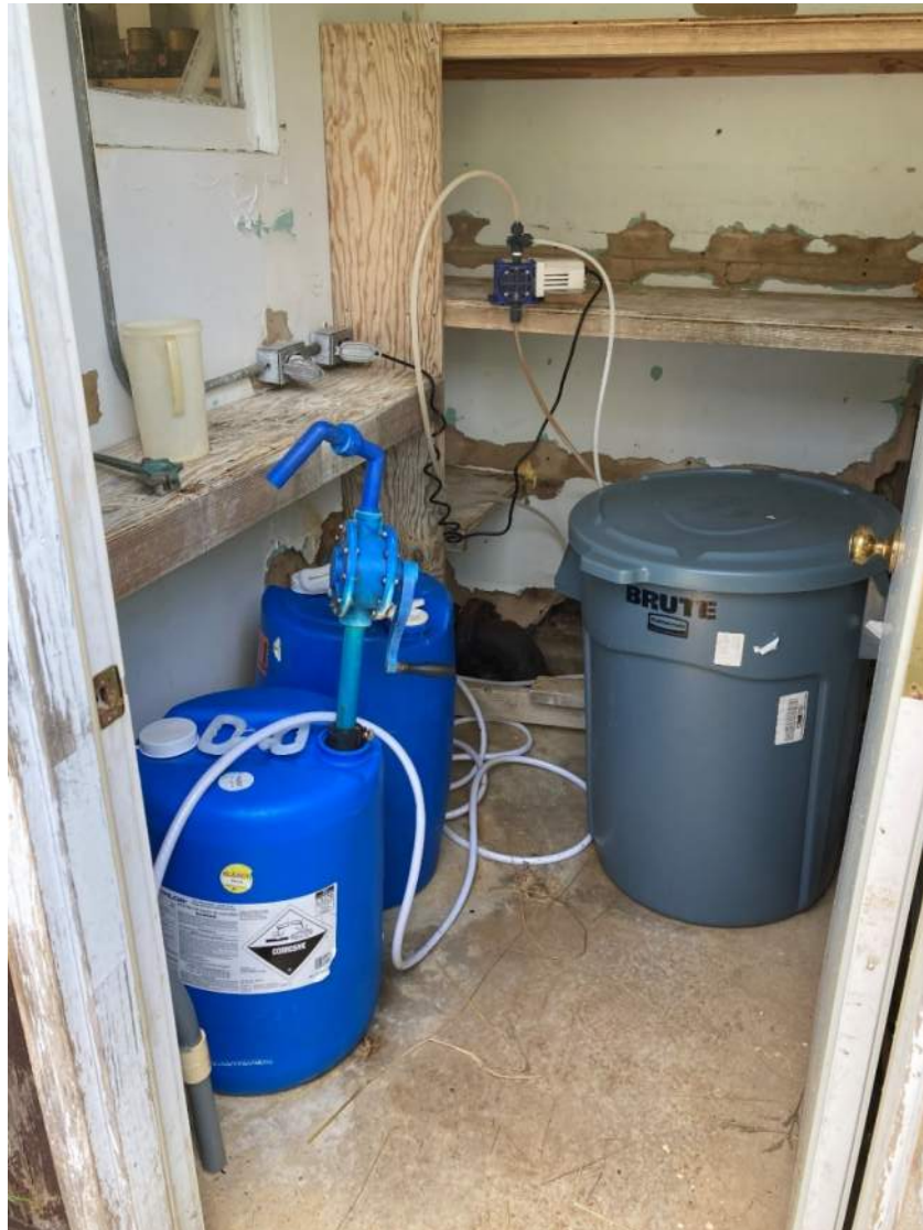
Figure 4-4 Chlorine Dosing System
