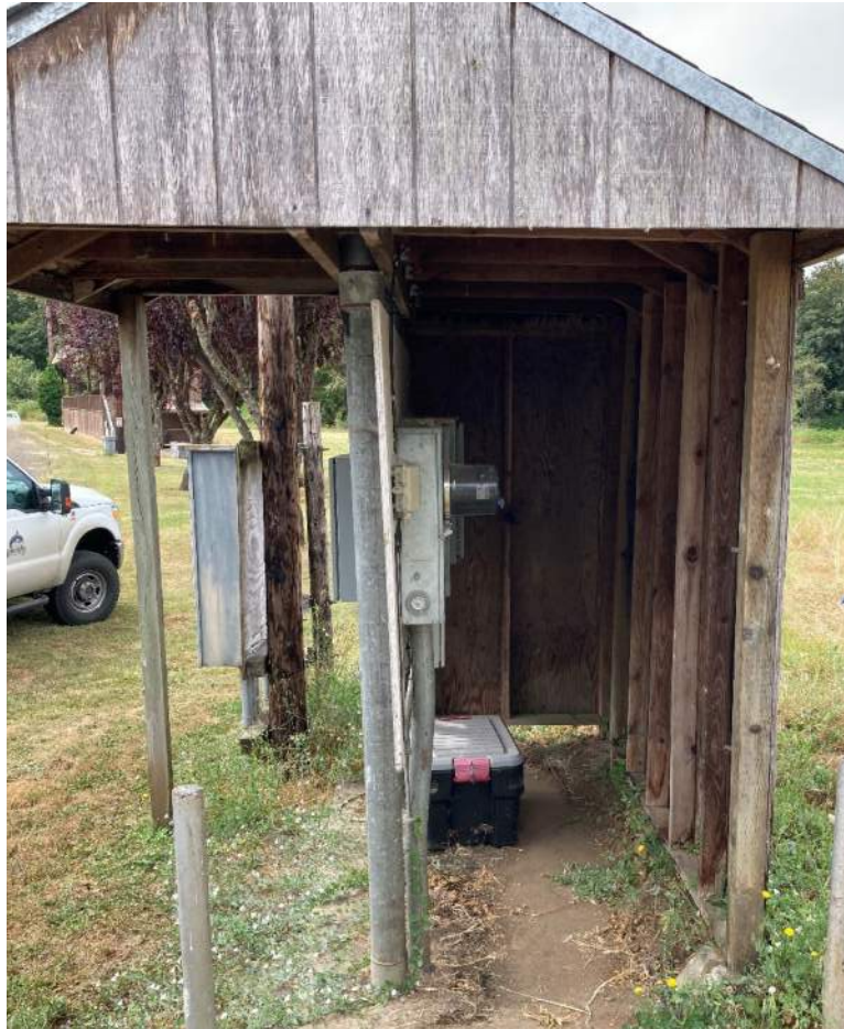
Figure 3-3 Lift Station Electrical and Controls Enclosure
