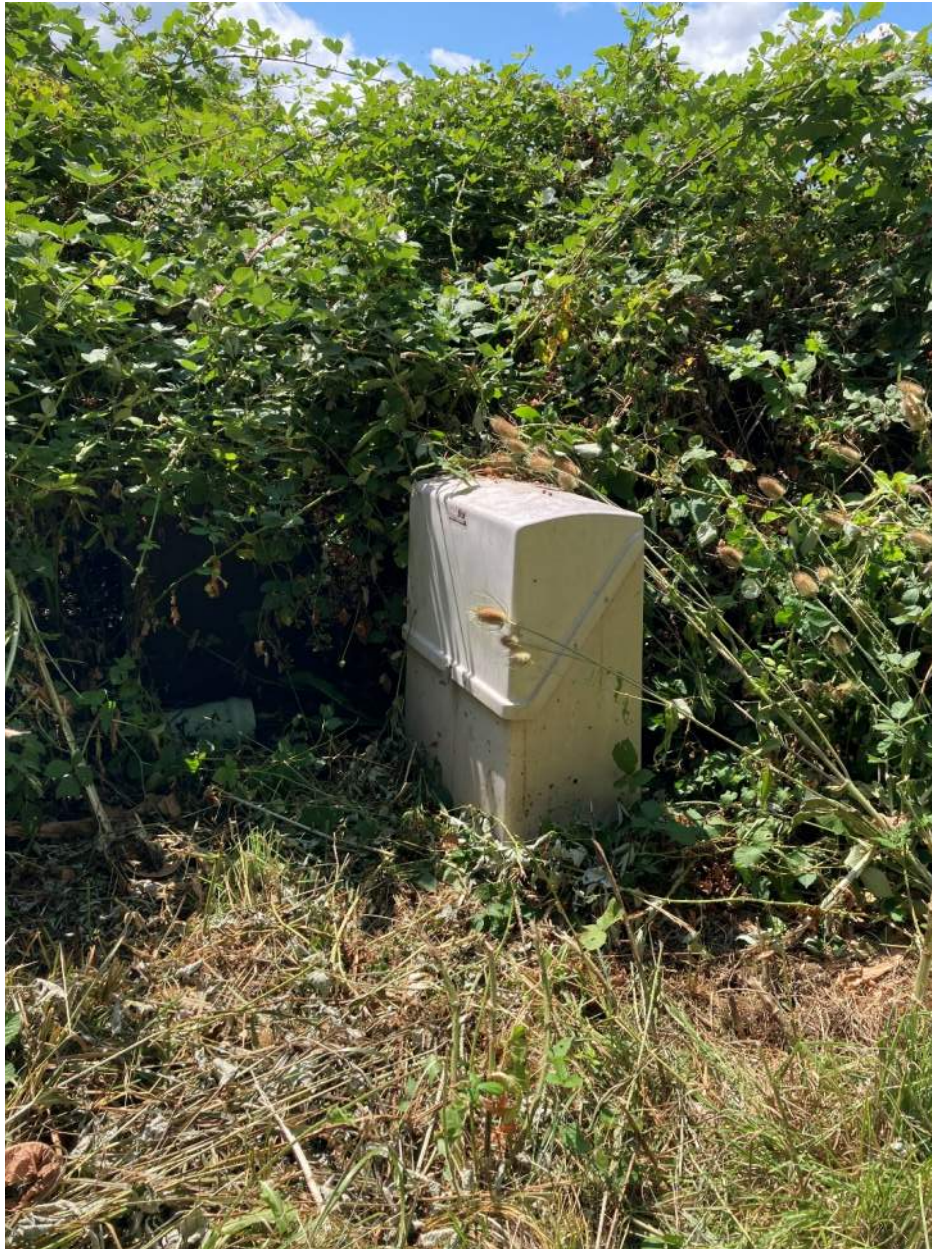
Figure 4-2 One of Two Wellheads Located Adjacent to the Wellhouse
