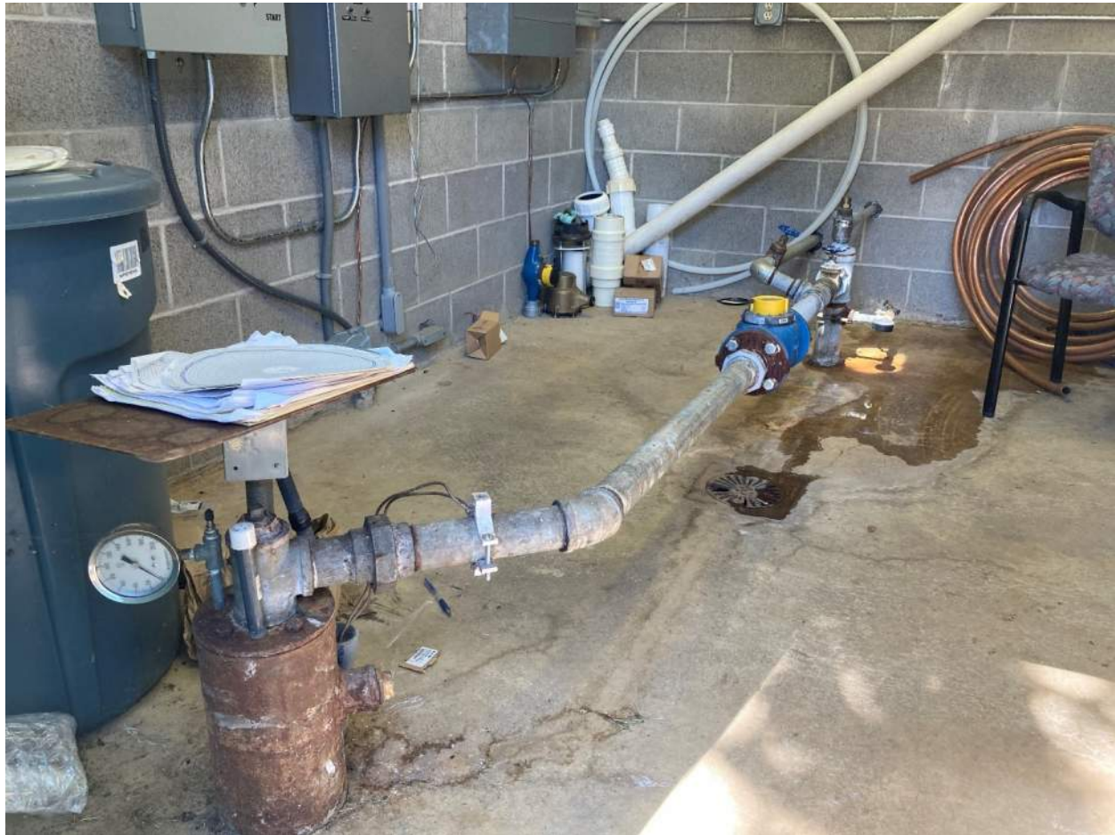
Figure 6-3 Well 2 Wellhead and Flowmeter
