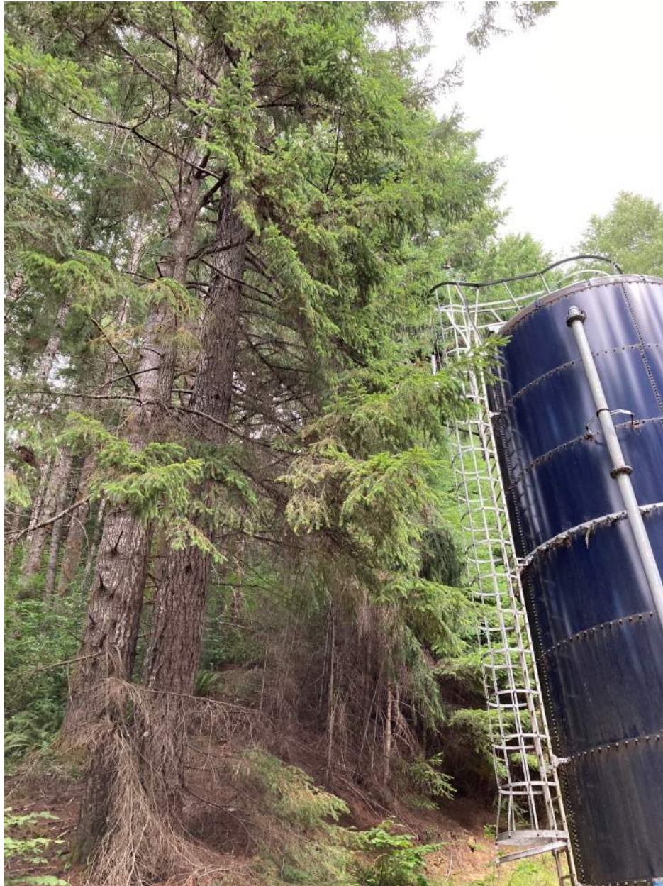
Figure 4-6 Vegetation Overhanging Bolted Steel Storage Tank
