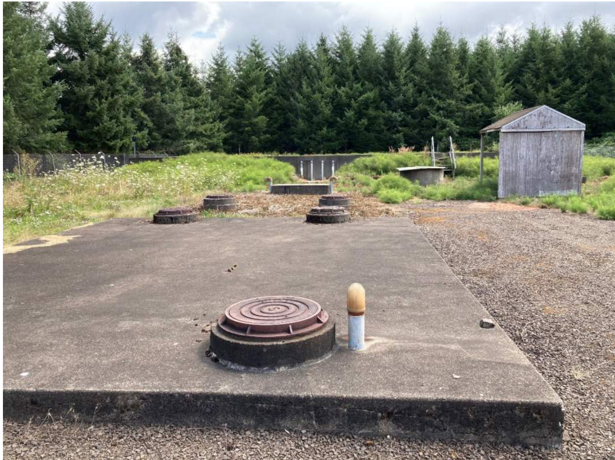
Figure 3-4 Septic Tank in Foreground, Wooden Structure Housing Controls
