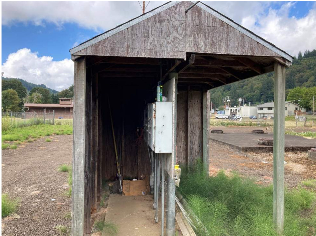
Figure 3-7 Electrical Equipment and Controls Structure
