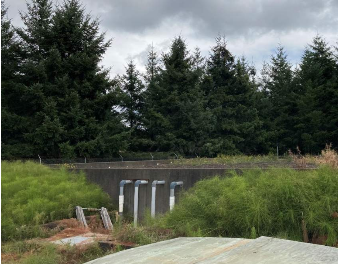
Figure 3-5 Recirculating Gravel Filter Basin with PVC Piping, Wooden Cover to Splitter Box in Foreground
