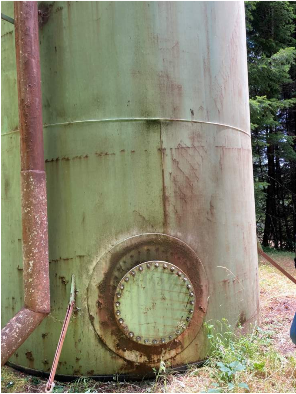
Figure 4-5 Access Hatch and Pitting on Welded Steel Storage Tank
