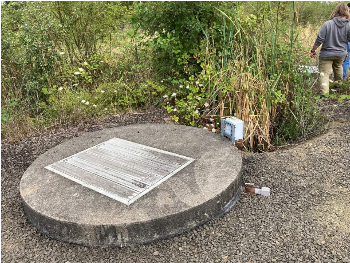
Figure 2-2 Influent Pump Station (In Foreground) and Meter Vault
