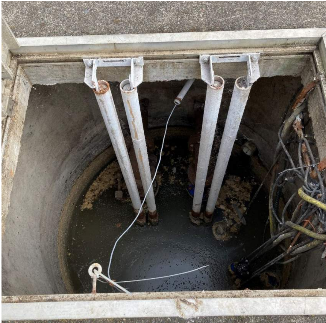
Figure 2-3 Influent Pump Station Interior
